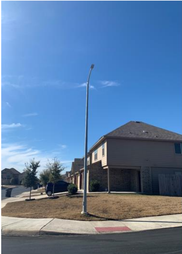
Existing CPS Energy Pole
