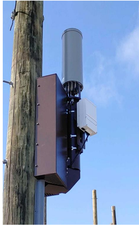
CPS Wood Pole "BEFORE"
