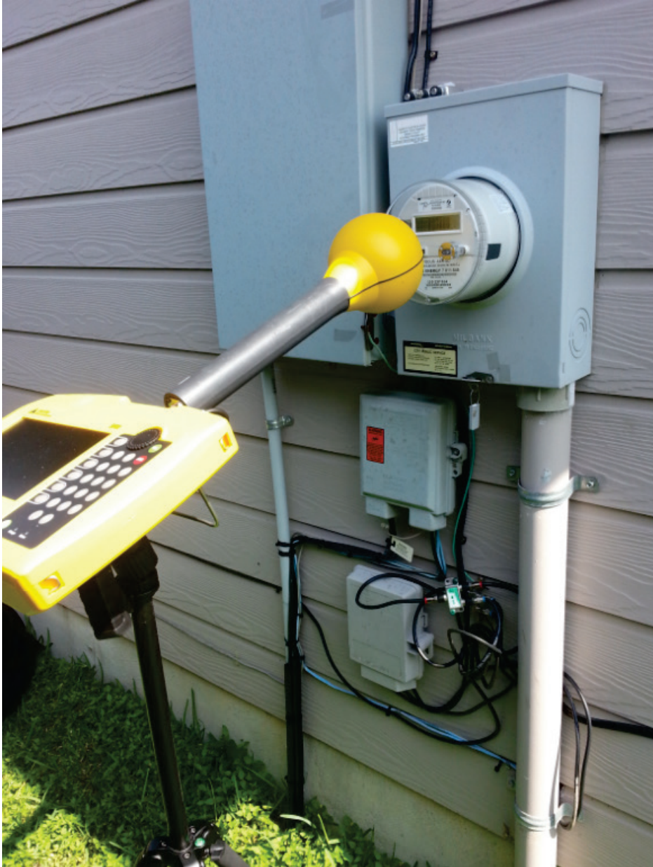
Figure B-3 Measurements near the meter in a residential installation
