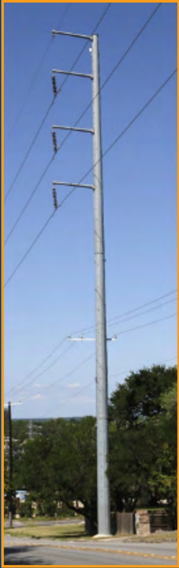
Single Circuit Structure
