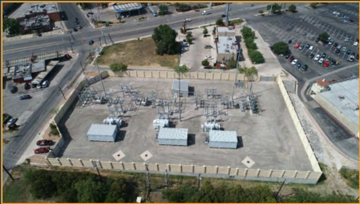
Exeter Substation – Typical Air Insulated Substation (AIS)
