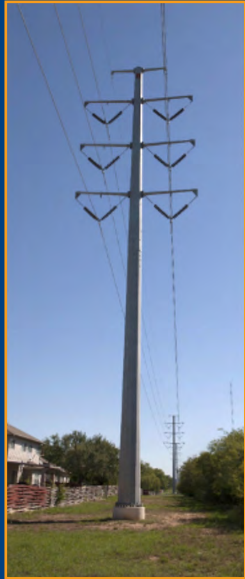
Double Circuit Structure
