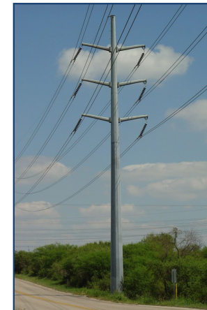
Solid Pole Structure
