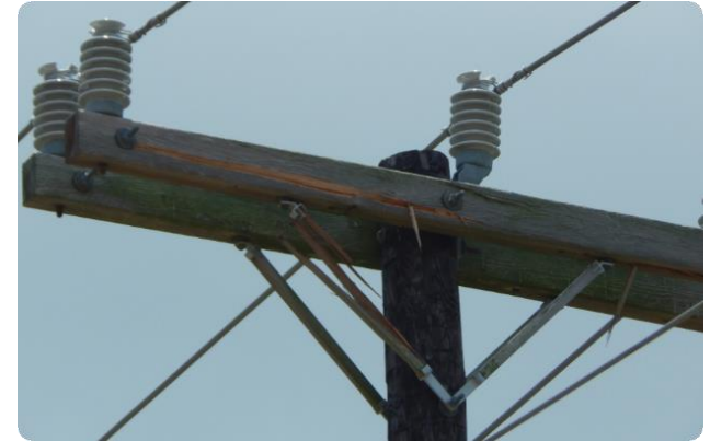
Lightning – damaged cross arm
