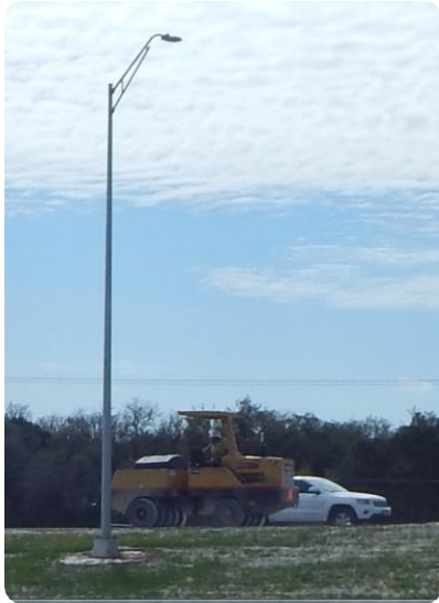
TXDOT Light Pole Installed Where Contact With Powerlines Occurred During High Winds. IH10 & Ranchland View
