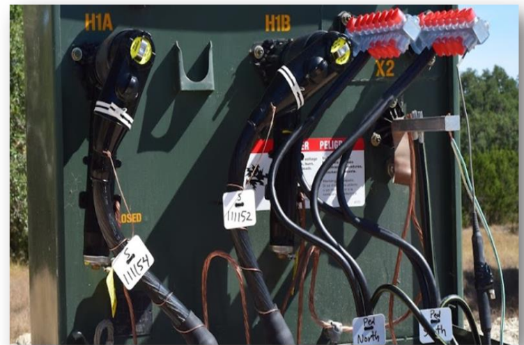
Terminated Cable for New Pad-Mount Transformer
